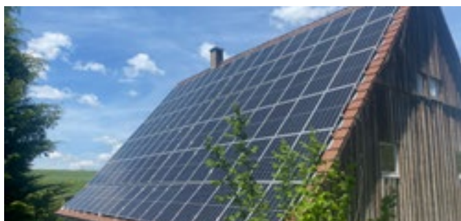
Private Anlage | Bad Waldsee 29,9 kWp
