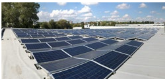
Helios Ventilatoren | Villingen-Schwenningen 199 kWp
